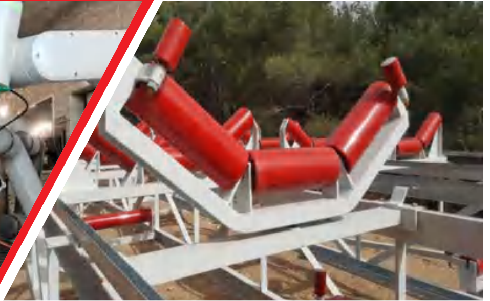
KOLİN TERMİK SANTRAL KOLIN THERMAL POWER PLANT
